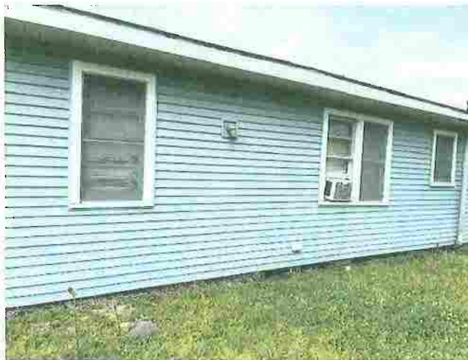
Picture taken April 12, 2023; AC window unit not properly installed allowing moisture into the interior will lead to rot and deterioration of the surrounding area.
