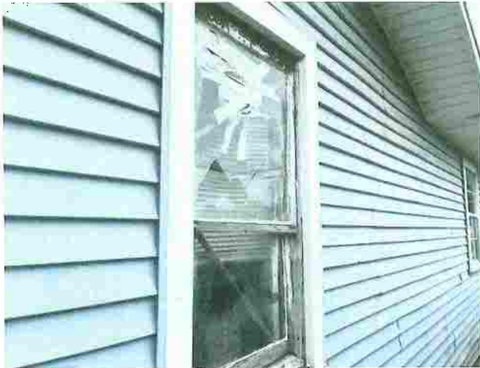
Picture taken April 12, 2023; window broken causing safety hazard and exposing the interior to the elements causing the sill and framing to rot.
