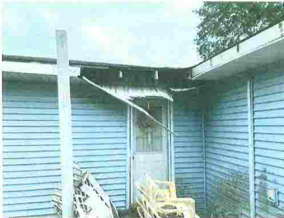
Picture taken April 12, 2023; Roofing trim, fascia, and boxing damaged with sections falling off exposing roofing supports to the elements and allowing moisture into the interior, exterior siding covered with algae and mildew.
