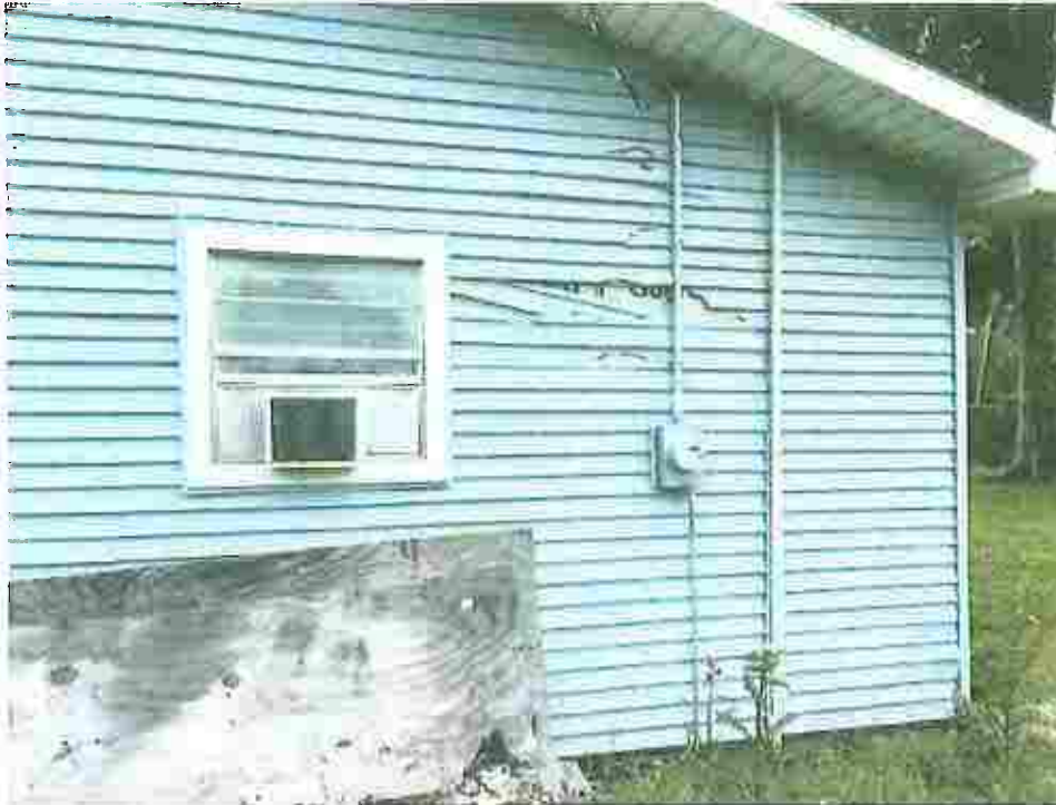
Picture taken April 12, 2023; exterior siding damaged exposing weather proofing underneath, AC window unit blocking emergency means of egress.
