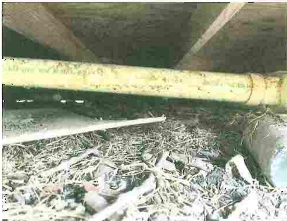
Picture taken April 13, 2023; sewer lines not properly anchored.
