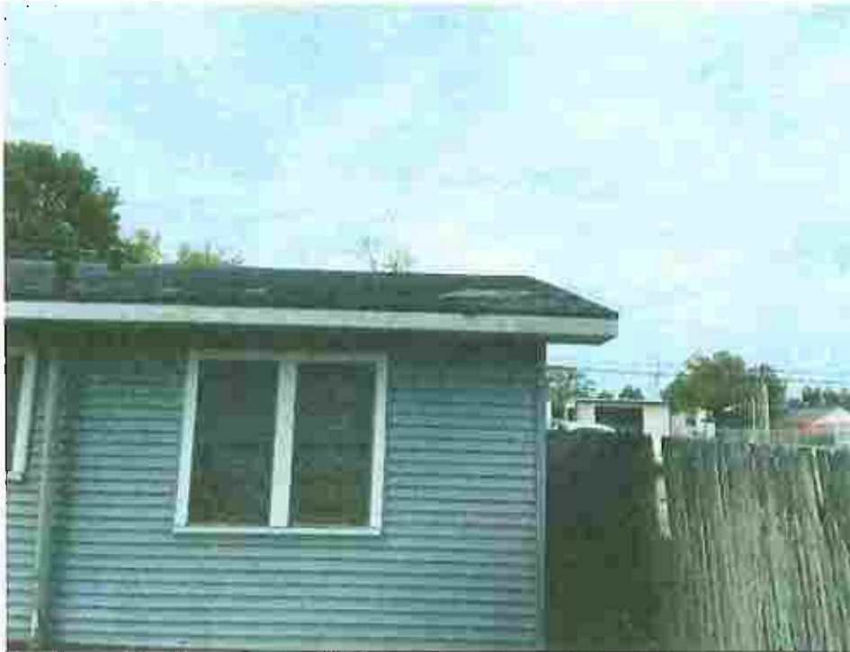
Picture taken April 12, 2023; roofing shingles damaged allowing moisture into the interior will lead to rot and deterioration.
