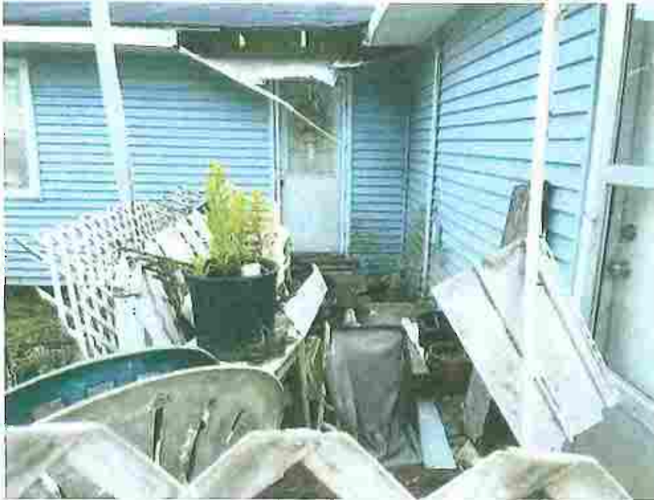
Picture taken April 12, 2023; Roofing trim, fascia, and boxing damaged with sections falling off exposing roofing supports to the elements and allowing moisture into the interior, exterior siding covered with algae and mildew, rubbish and debris piled outside of residence causing blighting and providing habitat for pest vermin.
