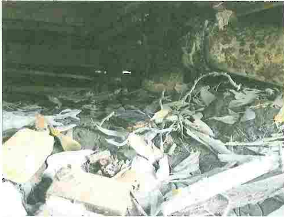
Picture taken April 13, 2023; sewer line broken allowing raw sewer to run onto the ground causing health hazard.
