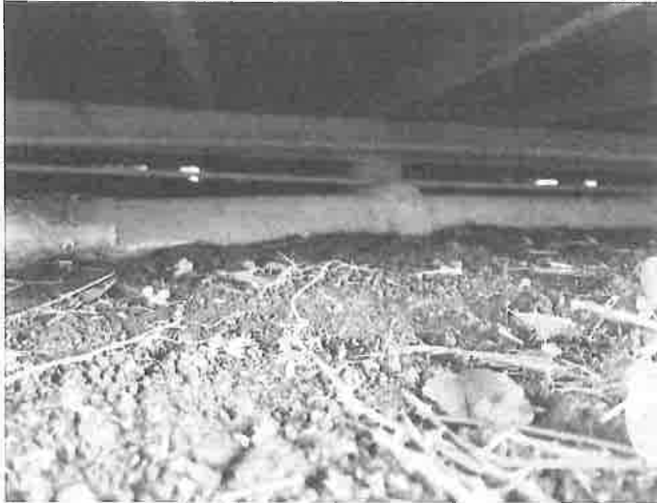
Picture taken April 13, 2023; plumbing lines not properly anchored.
