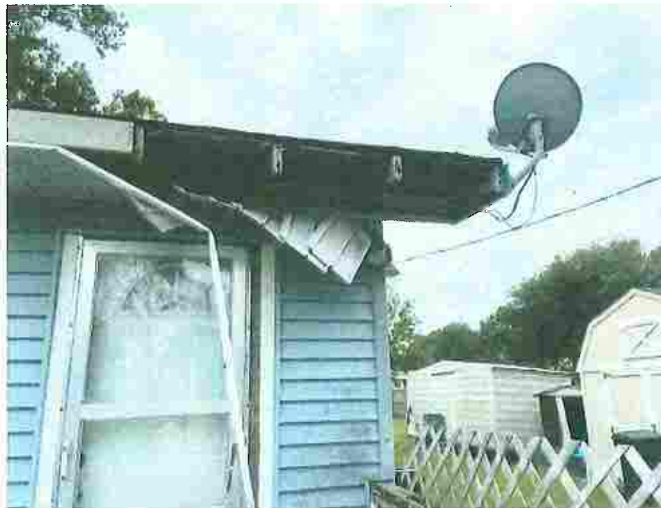
Picture taken April 12, 2023; Roofing trim, fascia, and boxing damaged with sections falling off exposing roofing supports to the elements and allowing moisture into the interior, exterior siding covered with algae and mildew.
