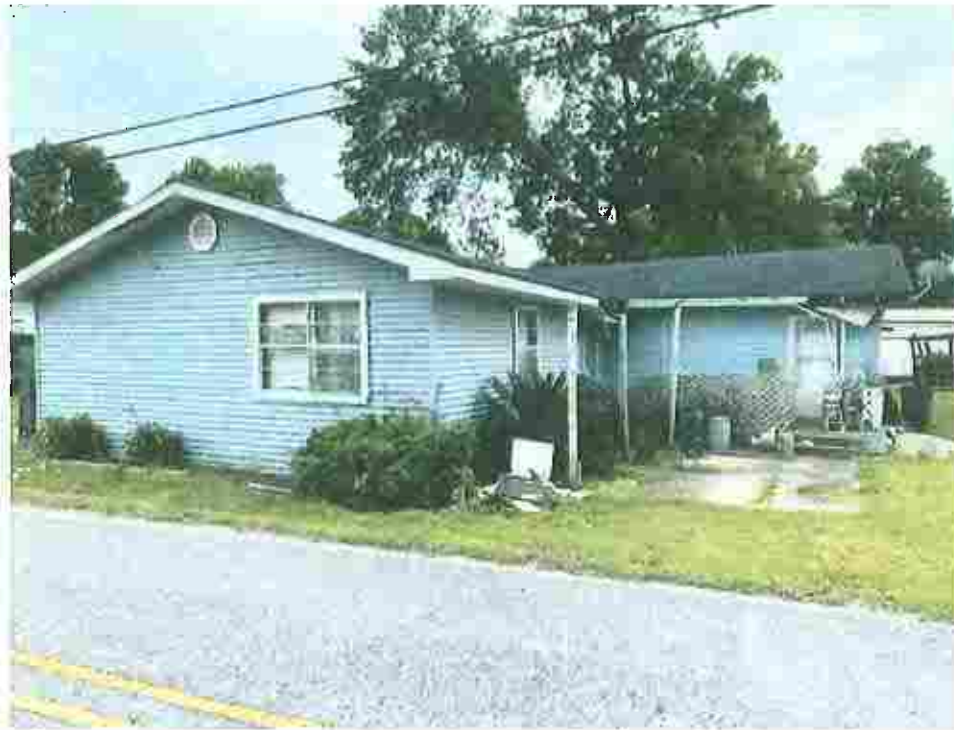
Picture taken April 12, 2023; Roofing trim, fascia, and boxing damaged with sections falling off exposing roofing supports to the elements and allowing moisture into the interior.
