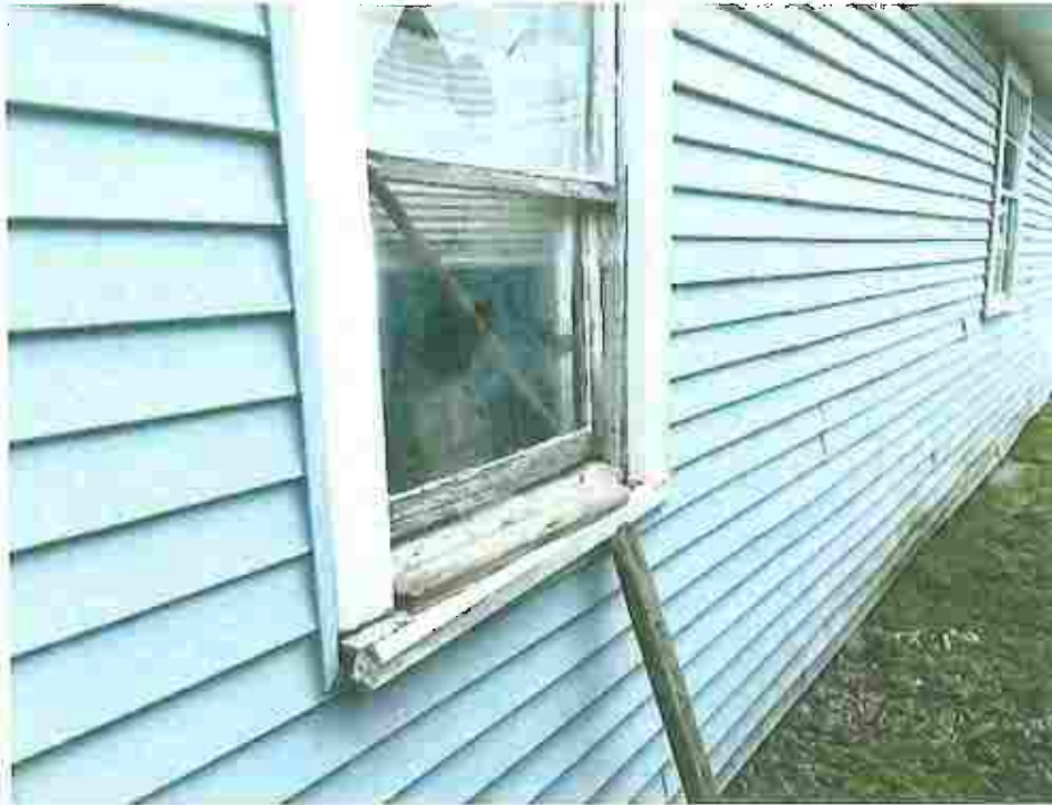
Picture taken April 12, 2023; window broken causing safety hazard and exposing the interior to the elements causing the sill and framing to rot.
