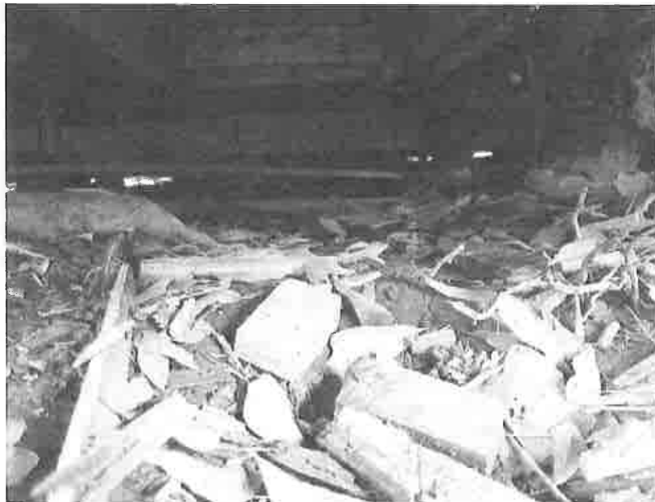
Picture taken April 13, 2023; sewer line broken allowing raw sewer to run onto the ground causing health hazard, foundation settled causing support beams and floor joist to not be attached.
