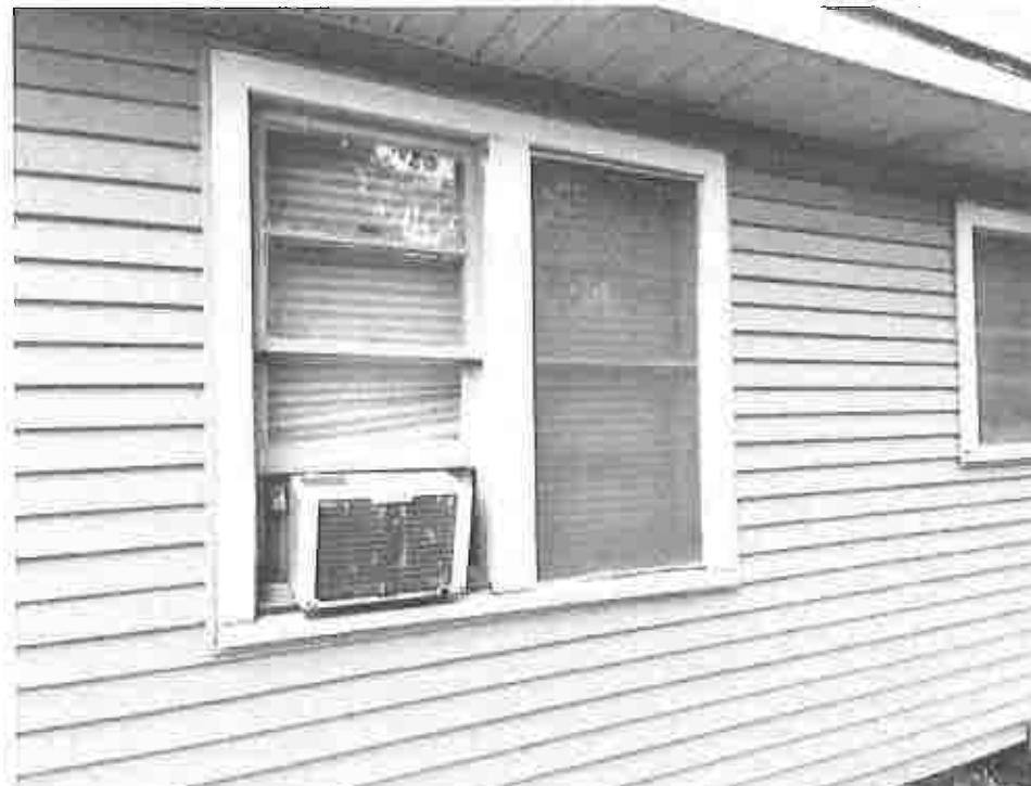
Picture taken April 12, 2023; AC window unit not properly installed allowing moisture into the interior will lead to rot and deterioration of the surrounding area.
