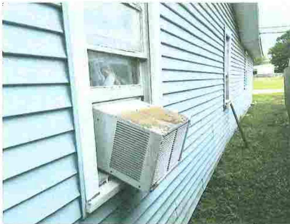
Picture taken April 12, 2023; AC window unit blocking means of egress.
