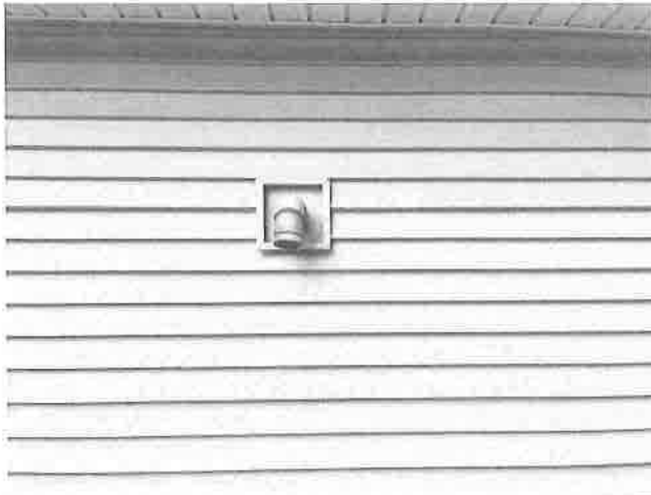
Picture taken April 12, 2023; heater vent line not code compliant.
