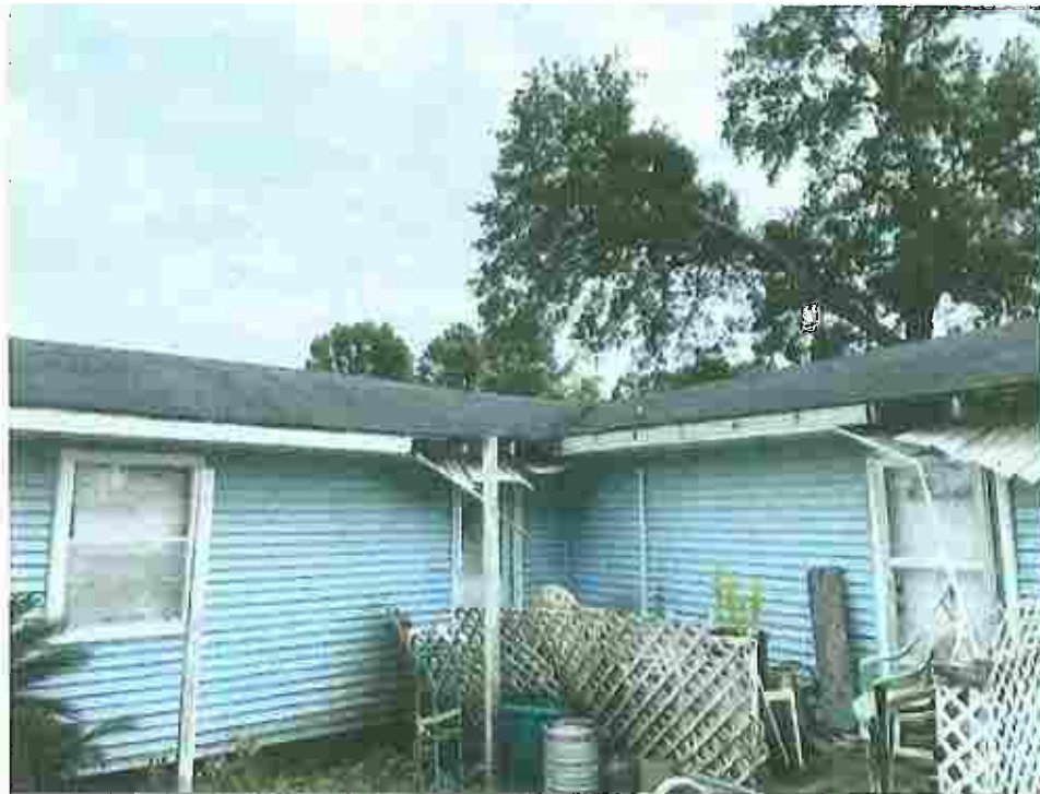
Picture taken April 12, 2023; Roofing trim, fascia, and boxing damaged with sections falling off exposing roofing supports to the elements and allowing moisture into the interior.
